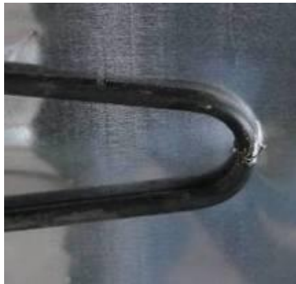
Absorber pipe fixed to backing plate with gal. wire
