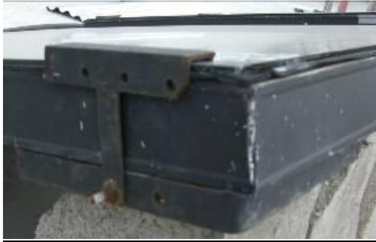
Top of collector brackets
