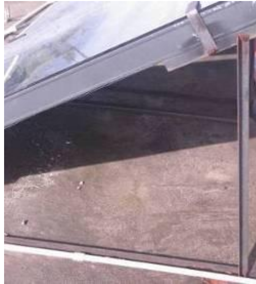
MS1 A-frame solar panel support structures (Nueva Alianza)
